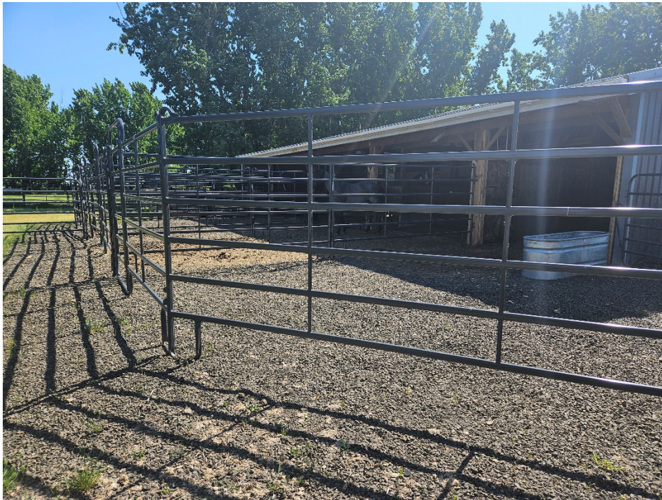
After: Project completion with hard rock surface area, gutters and new paddock fencing
