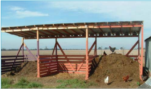
The building of this composting structure near Finley Wildlife Refuge was inspired during the Horses & Mud workshop with OSU Extension Small Farms agent, Melissa Fery. Building materials were funded by an OWEB Small Grant. Proper manure management improves nutrient cycling and protects water quality.
