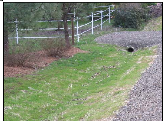
After: Graded slope and erosion control fabric permit grass to grow and protect the site from further erosion.
