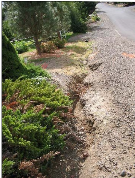
Before: Soil erosion along the ditch had occurred after several large storms.
