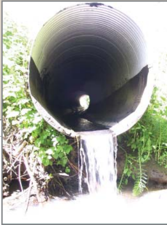
The perched Blair Creek culvert hindered fish passage prior to replacement.
